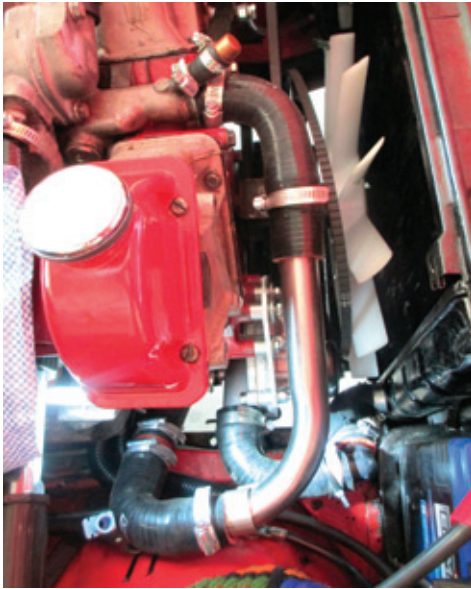
External belt-driven pump in place with original lower hose connections to original radiator - Image: Tanya Duke
